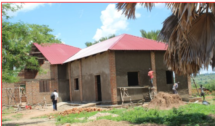
The latest view of the PLC as the workers “plaster” the outside walls. The project was made possible by a donation from a St. Roch parish-ioner, St. Barnabas Parish and the Christians of Aripea Parish.
