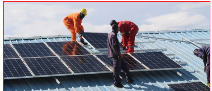
Our chief technician, Enguma Samson, and his team position solar panels on the roof of the administration building at Radio Pacis.
