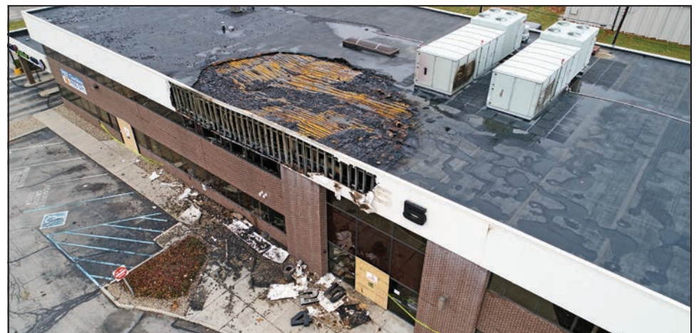
This overhead drone shot on Dec. 1 shows damage to an office building on the northwest side of Indianapolis that occurred late on Nov. 30. Two pro-life organizations were affected. 1st Choice for Women, which offers free peer-counseling, pregnancy tests and ultrasounds, is located below the second-floor area where the fire started. Magnificat Family Medicine is located on the second floor to the right of the fire damage. (Submitted photo by Colin Landberg/Pike Township Fire Department)
