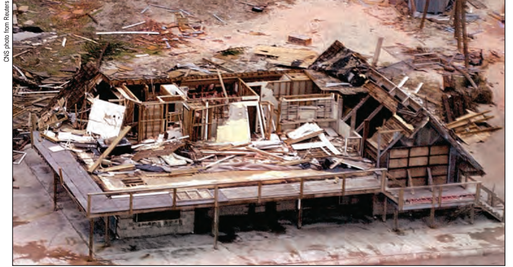
A house along the coast lies destroyed after Hurricane Jeanne hit Vero Beach, Fla., Sept. 26. Adults often wonder how much insurance they need. In the case of home insurance, the conventional wisdom is that a house should be insured for its replacement value.
