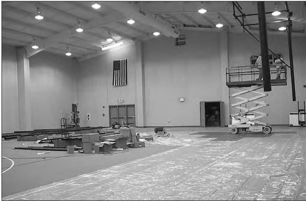
Workers put up the basketball goals in the new gymnasium at St. Michael Parish in Brookville. The gymnasium is part of a new parish activity center that also contains a cafeteria and kitchen, and is connected to St. Michael School.
